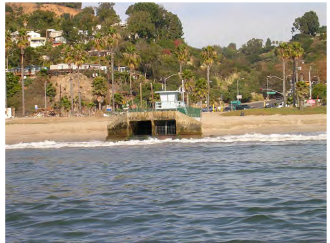
Los Angeles storm drain entering the ocean. (Photo credit: Phyllis Grifman, USC Sea Grant)
