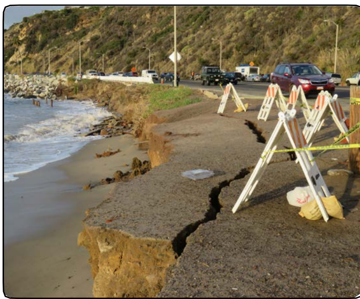
Erosion in Malibu from winter storms
