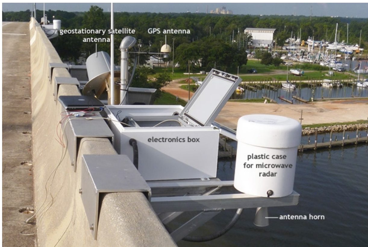
A microwave radar attached to a bridge over the Dog River in Alabama. The radar, encased in the white plastic housing in the foreground, sends a pulse of microwave energy down toward the water surface and listens for the echo. The higher the water, the quicker return echo. NOAA photo courtesy Morgan McHugh.
